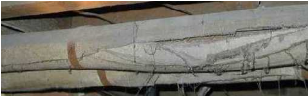
The above photo shows a typical asbestos insulated heating pipe found in older homes.
